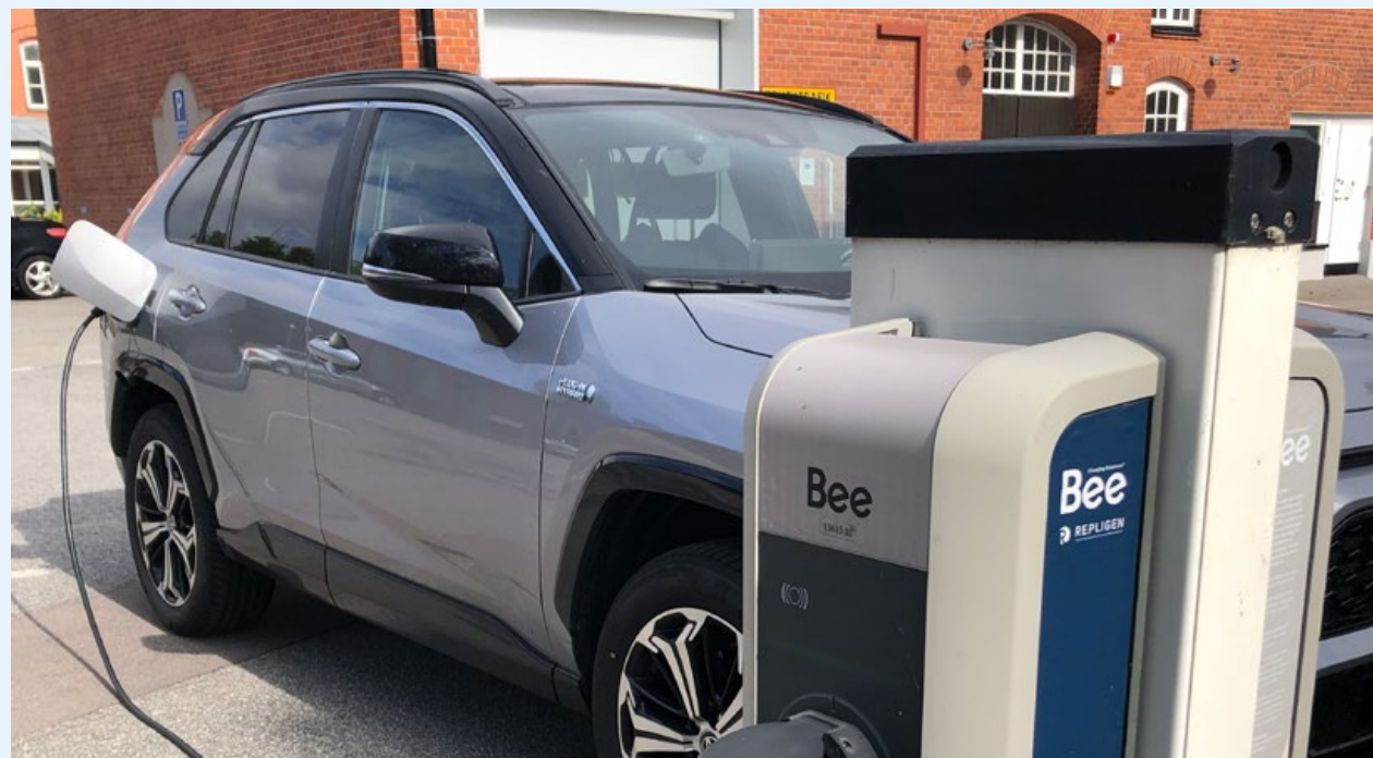
Electric car charging station in Lund.
